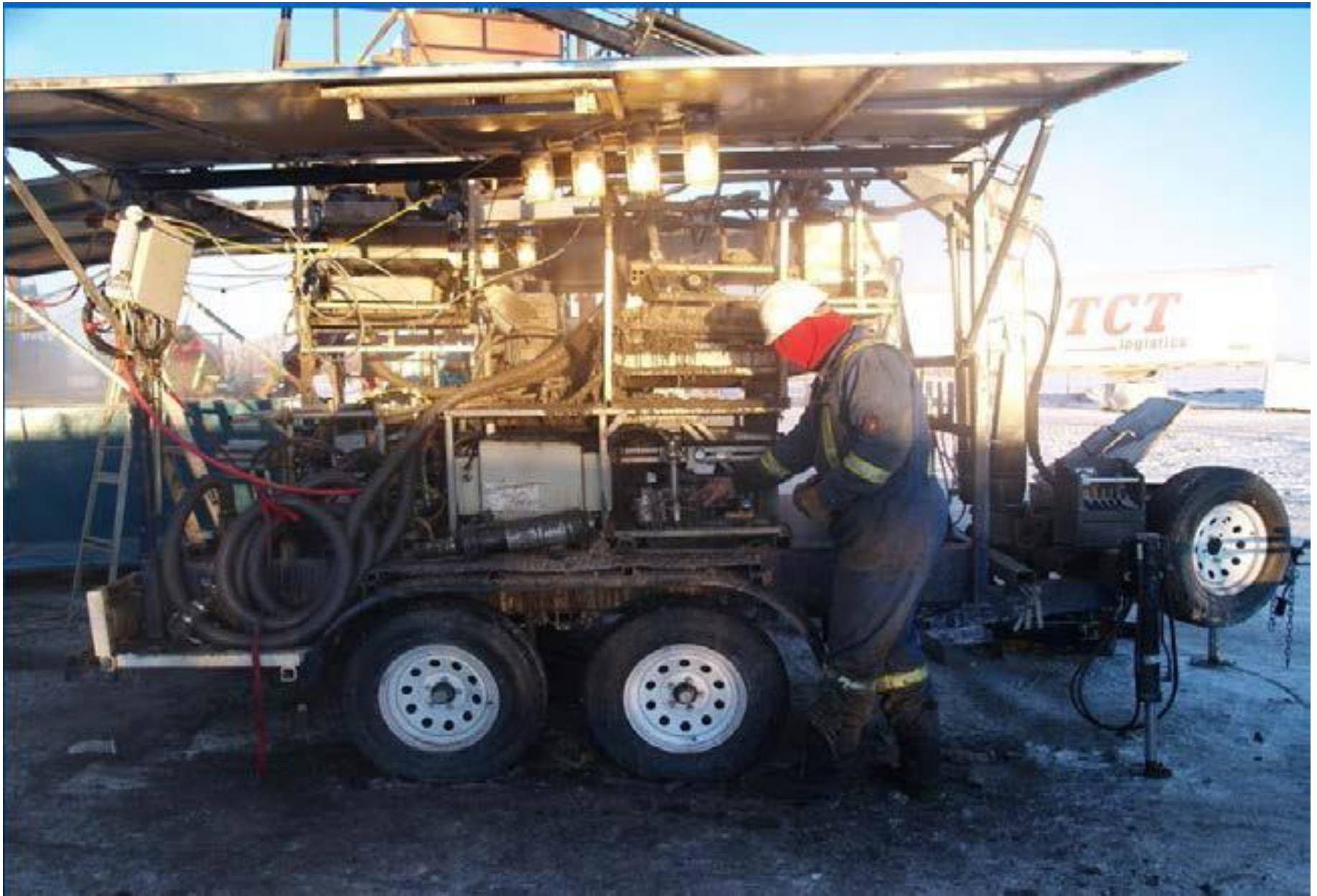
Figure 1. The OPAL system at the wellsite.
