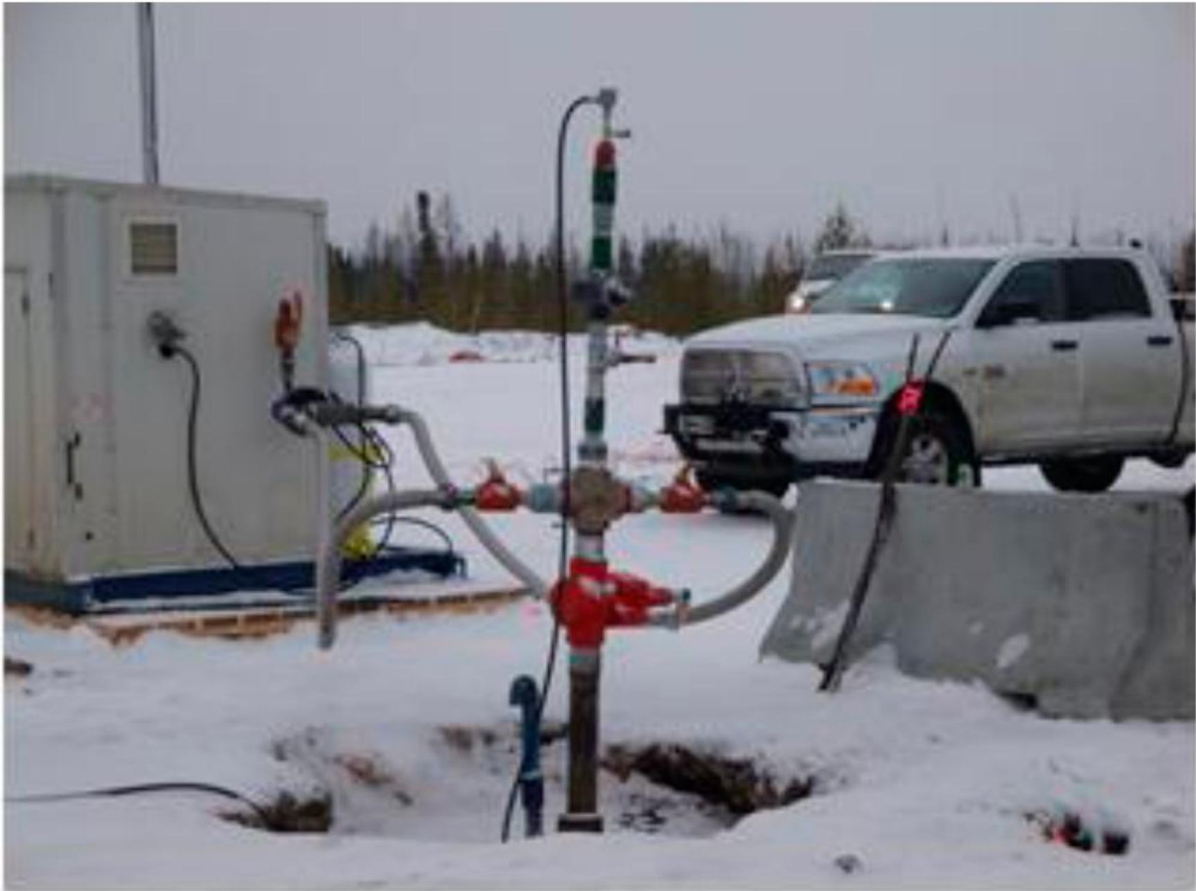
Figure 2. Air injection set up at the 02-27 location.
