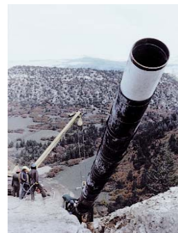
CO 2 transport (Cortez pipeline booster, USA)
