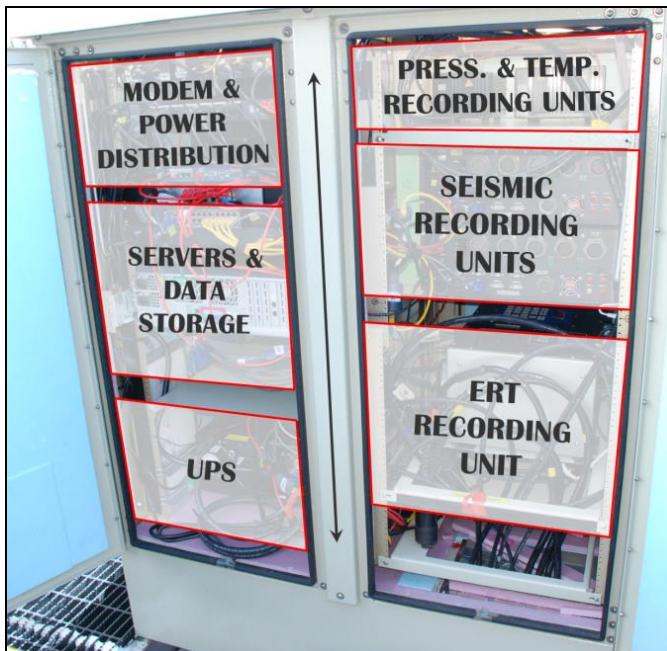
Figure 2: Schematic view of the instrument cabinet located close to the two observation wells at LDA. All instruments can be controlled through the Statoil network to record data throughout the year. In addition to recording instruments, the cabinet is equipped with data servers, an uninterruptible power supply (UPS), air conditioning and more. The arrow in the middle is approximately 1 meter.
