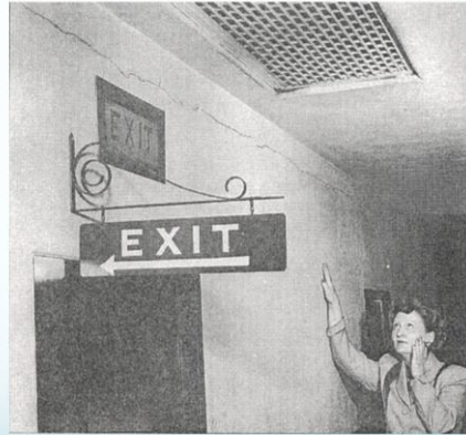
Crack in OKC State Building
